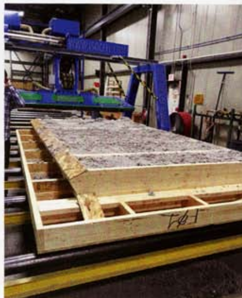
The Tektoniks production line turns out high-performance building components in a controlled environment where ice, snow and rain aren't factors. The Lovell, Maine, home was the first to be produced by the Bensonwood subsidiary.
